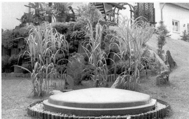
Fig 14 Installed RBC (CAT 2000)
