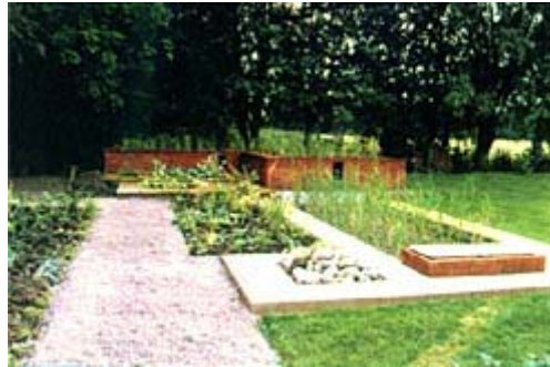
Fig.5 Unobtrusive complete horizontal and vertical reed bed sewage treatment system installed at a hotel and serving a population of 24.
